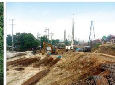
BANGLADESH Bangladesh SASEC Road Project(WP-01) Northwest Dhaka, Bangladesh L 18.9km, Road Repair, Improvement, and Extended Pavement(2 Lanes → 4 Lanes)
