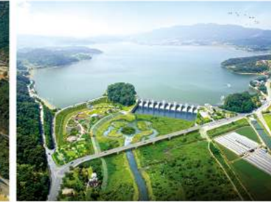
Yedang Reservoir Disaster Prevention Spillway Expansion Project [Agricultural Civil Works] Spillway Expansion, Maintenance Road and Waterside Park Construction
