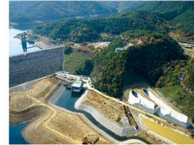
Juam Dam Emergency Spillway [Agricultural Civil Works] Tunnel-type WaterWay, D 12.8m, L 542m, 2 Girders
